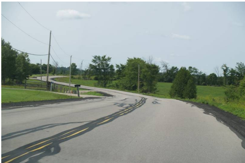
Figure 2.2 Obscured centerline pavement markings due to crack sealing (CR 10)
