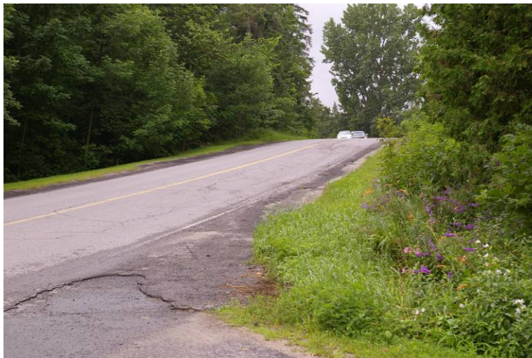
Figure 2.1 Inadequate sight lines of approaching eastbound traffic (CR 12 at Argyle Street)
