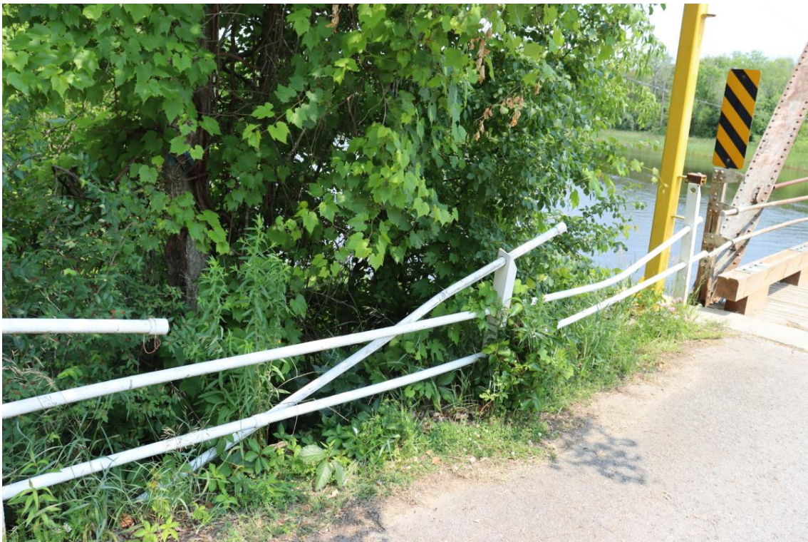
Figure 68: NW damaged approach railing
