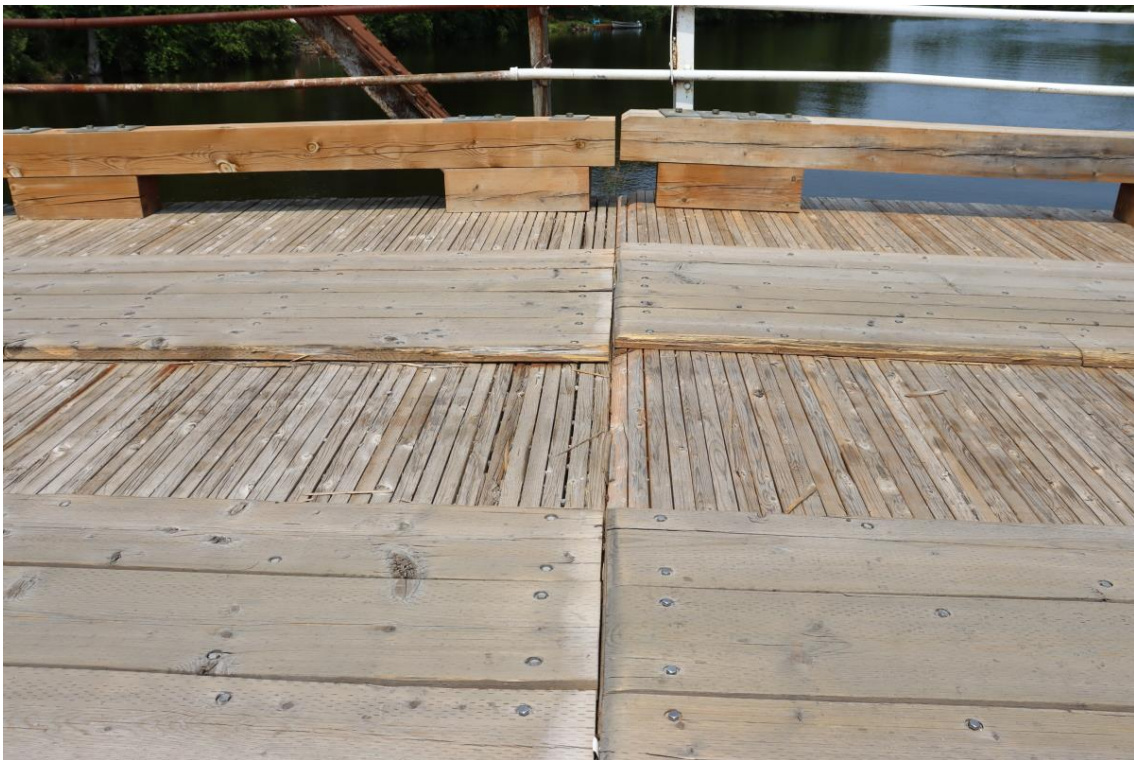
Figure 54: Grade change / bump over pier
