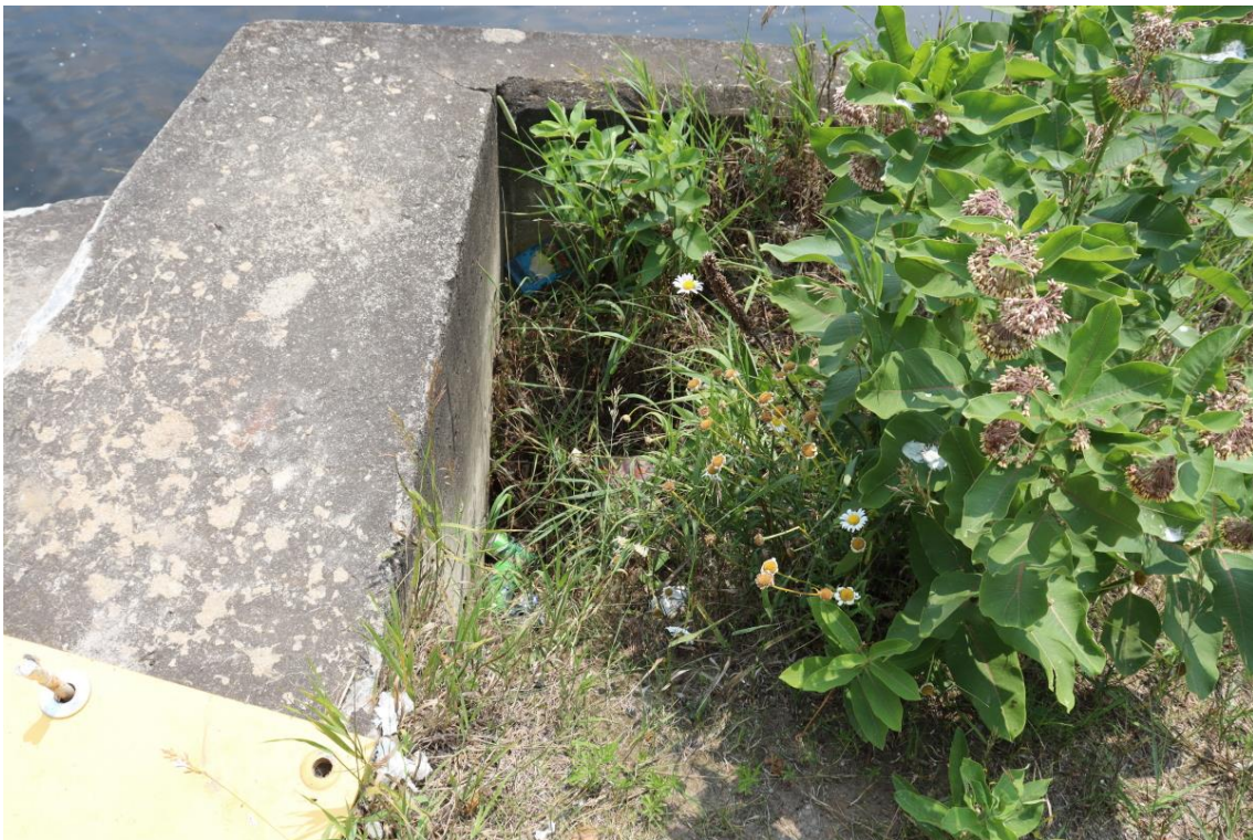
Figure 42: Sinkhole in SW corner
