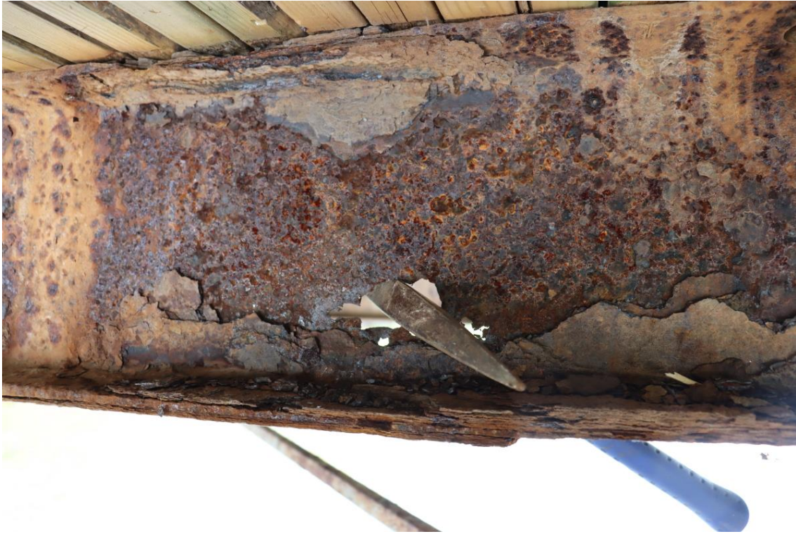
Figure 39: Stringer 3 perforation in bay 5
