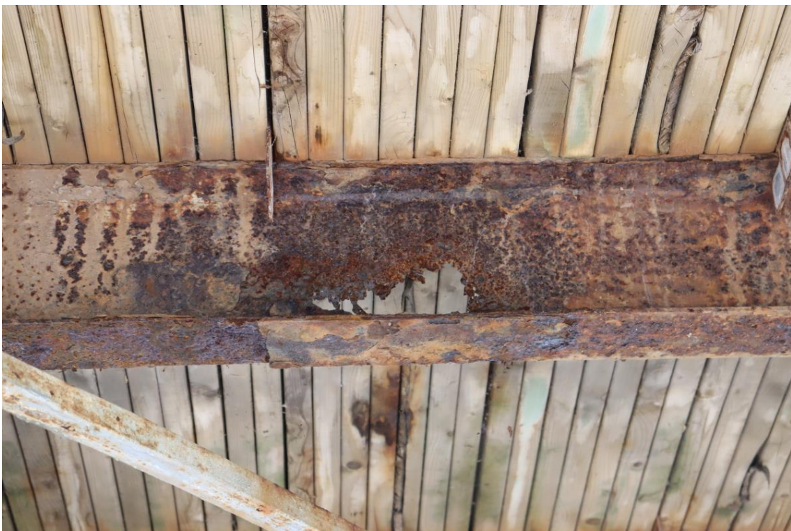
Figure 10: Stringer 2 perforation in bay 8
