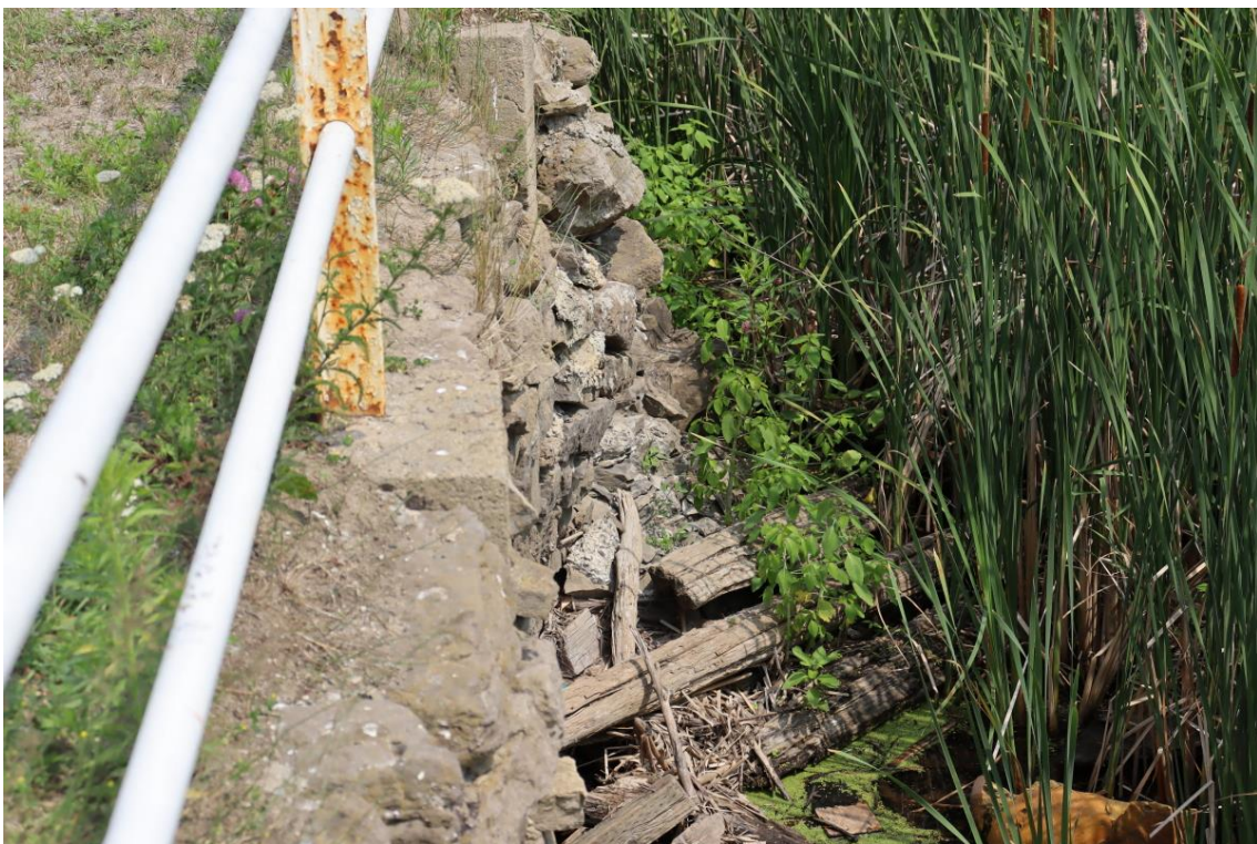
Figure 32: Bulging retaining wall in SE
