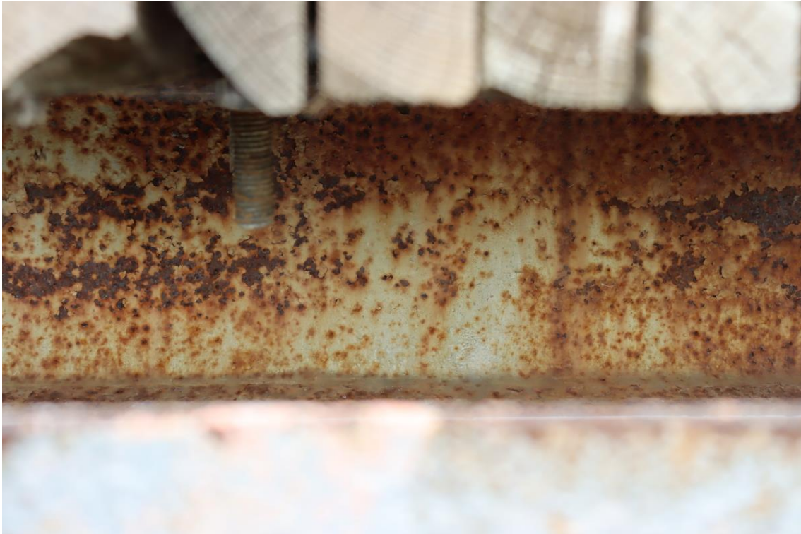
Figure 35: External stringer 1 condition Bay 6
