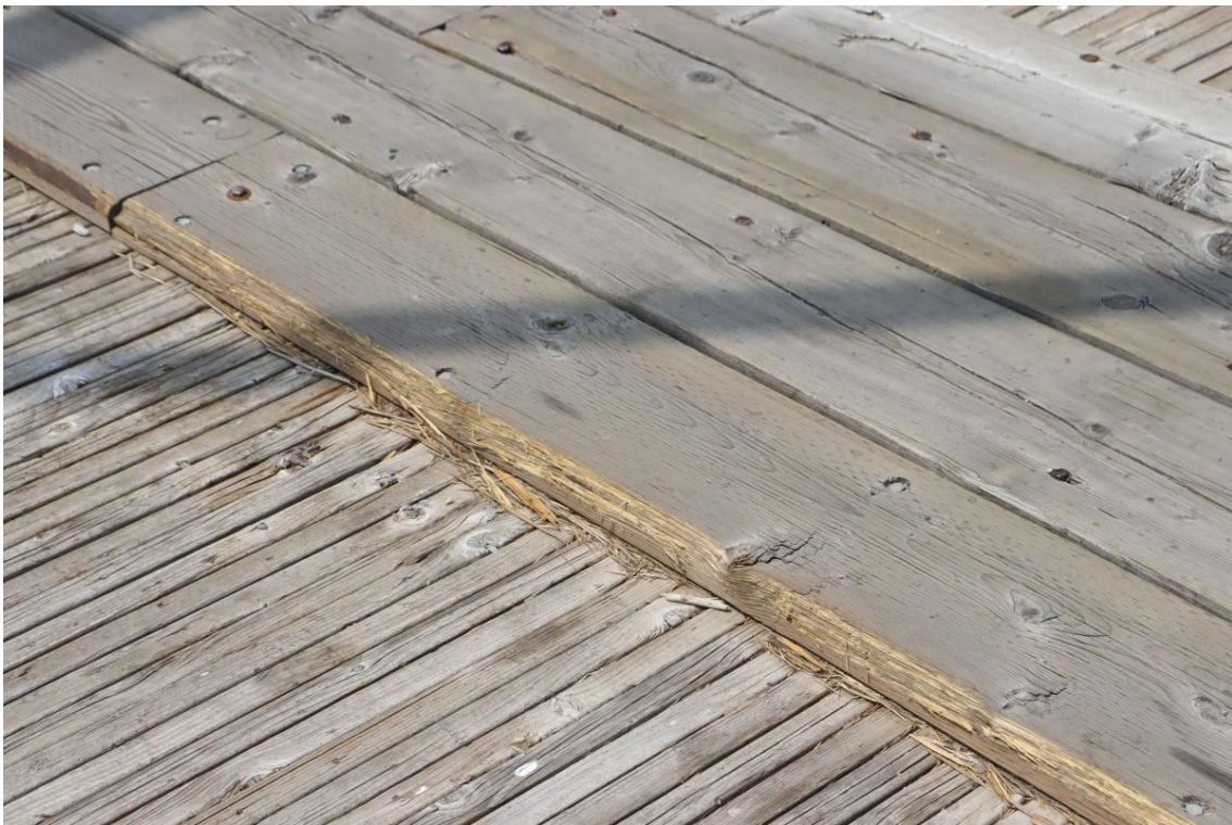
Figure 60: Damaged running boards
