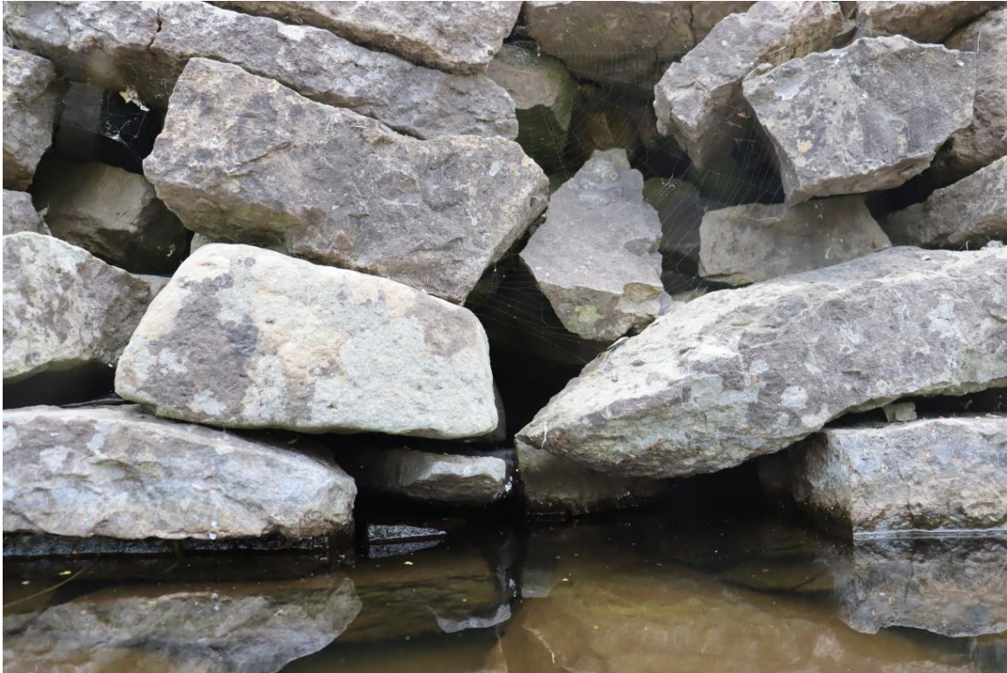
Figure 49: Blocked drainage opening through causeway
