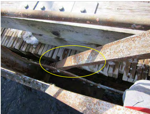
Photograph 6: Twisting of U2L3 (east truss) near L3.
