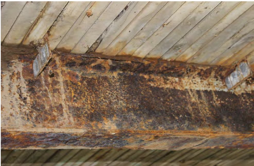
Image 10. North face of Stringer 4 between FB 7 & pier, severe thinning of top flange
