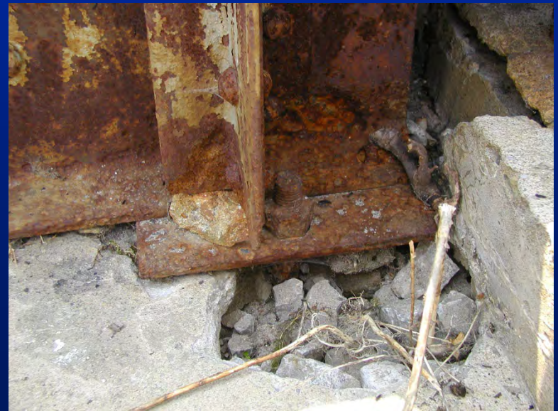
Undermining of south pier bearing
