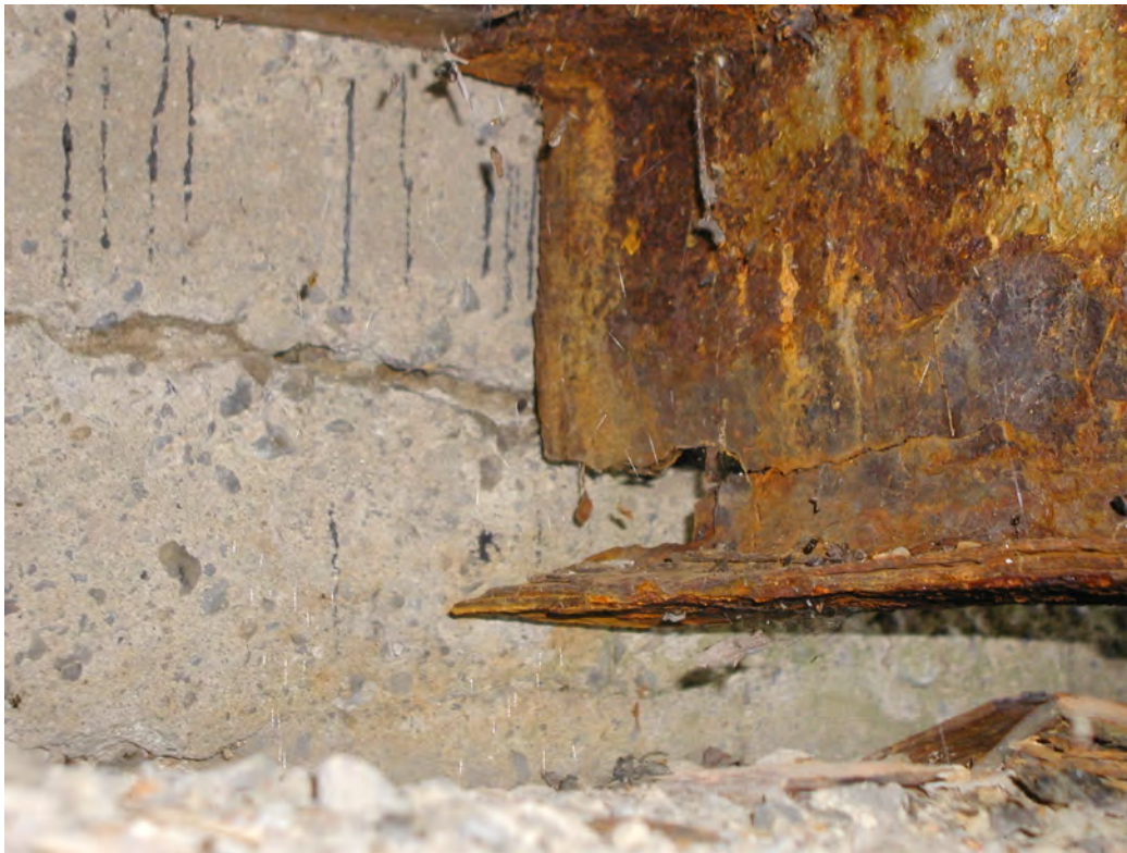
Photograph 20: Section loss and crack in web of exterior stringer, West Abutment.
