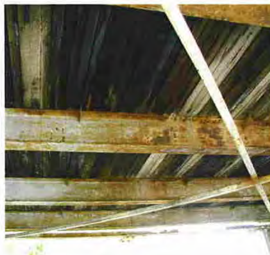
Photograph 5: Deterioration of the timber deck due to loss of creosote protection. Note the widespread light corrosion of the below-deck steel floor system.
