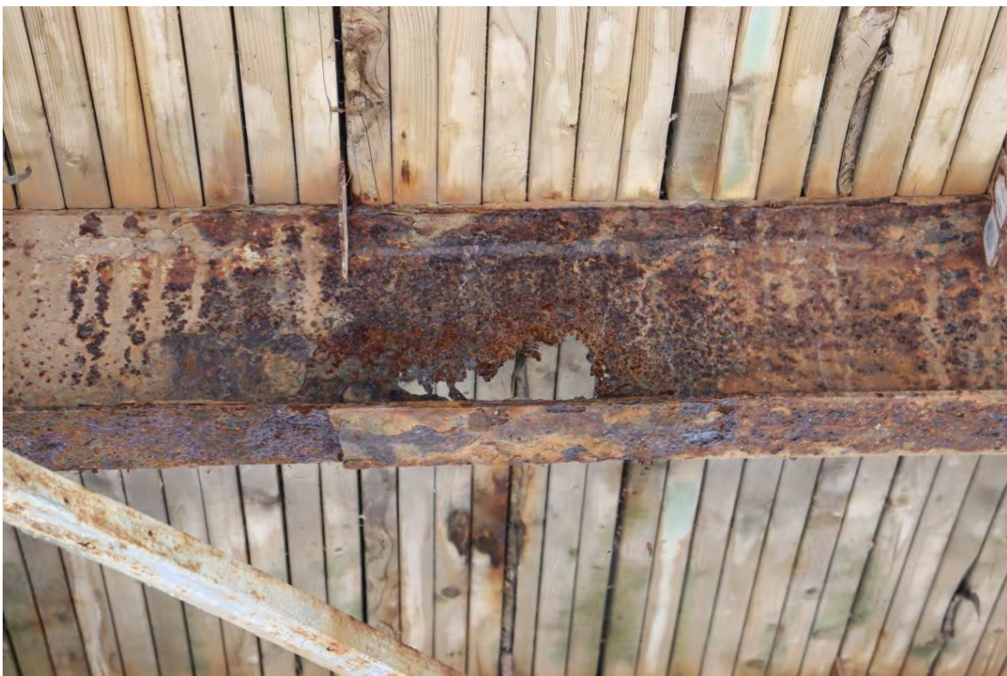
Figure 10: Stringer 2 perforation in bay 8
