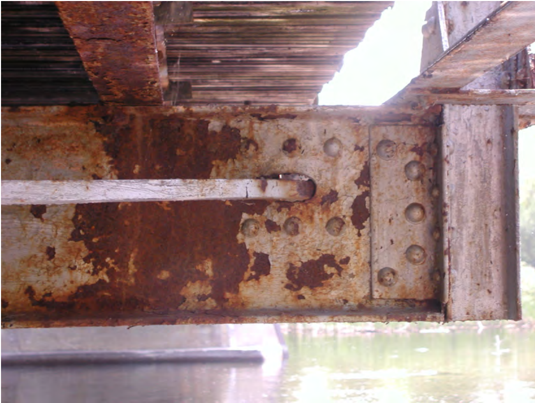
Photograph 15: Detail of cross-bracing as it passes through the web of the floorbeam.
