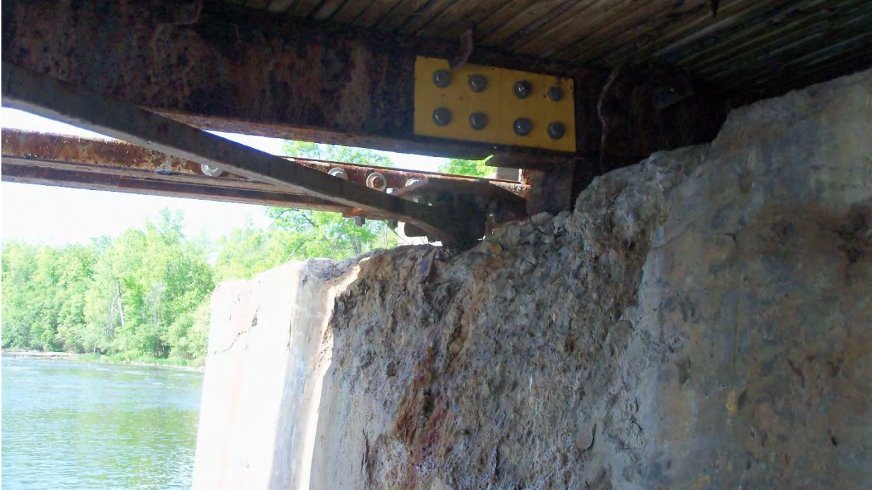
View showing severe spalling of abutment and replaced bolted end plates
