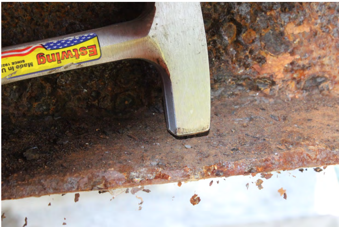
Image 4. Close up of Image 3. Rust dangling from spider webs
