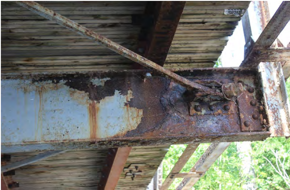
Image 2. North end of Floor Beam 1 (FB 1) with slab rust evident
