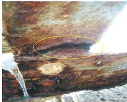
Photograph 3: Severe pitting of horizontal leg of bottom chord L0L1.
