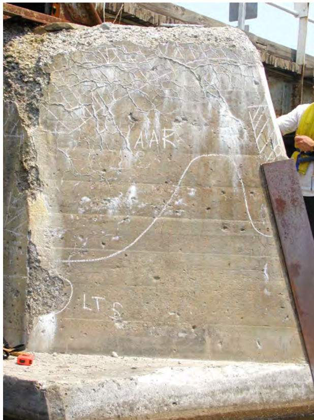
Photograph 28: Deterioration of west face of pier nosing. Note extensive deterioration and alkali-aggregate reaction. Condition of east face is similar.
