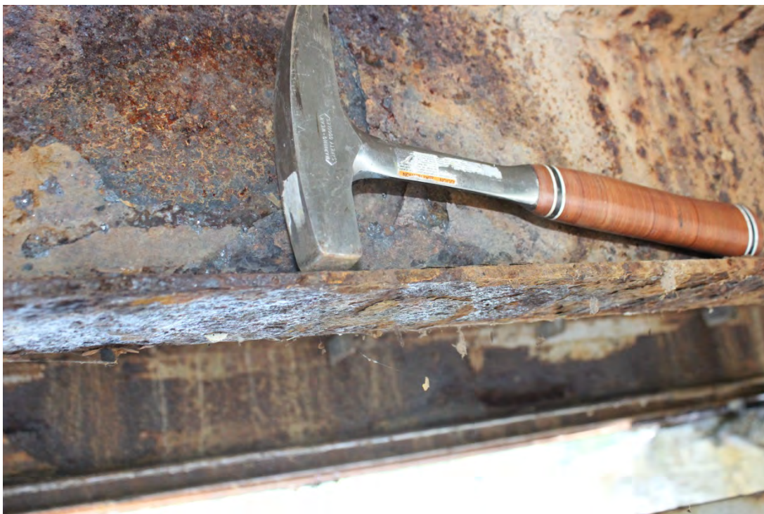
Image 6. Typical corrosion on stringers Bay 1
