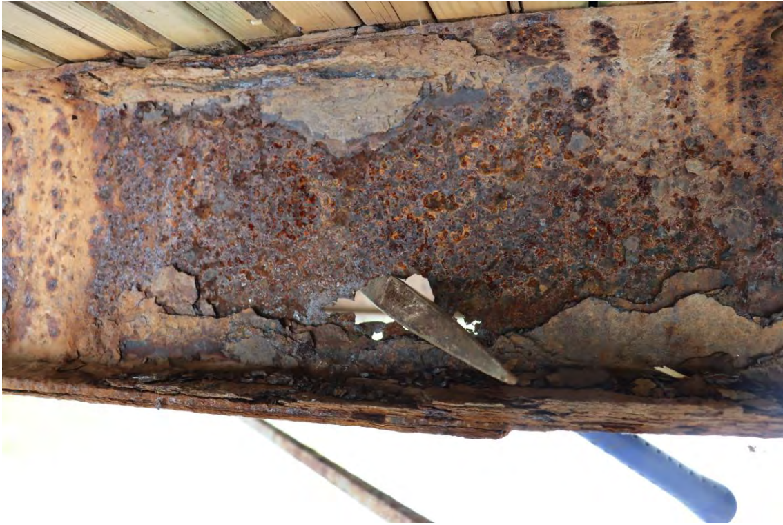
Figure 39: Stringer 3 perforation in bay 5
