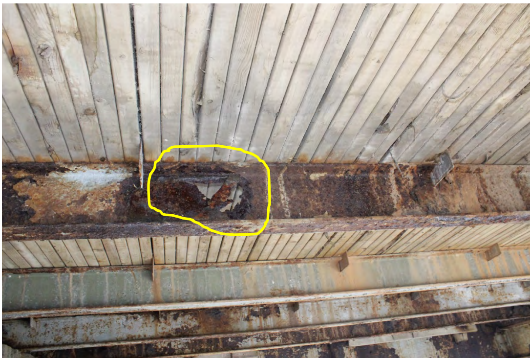
Image 12. Perforation of Approach Stringer 2 before probing
