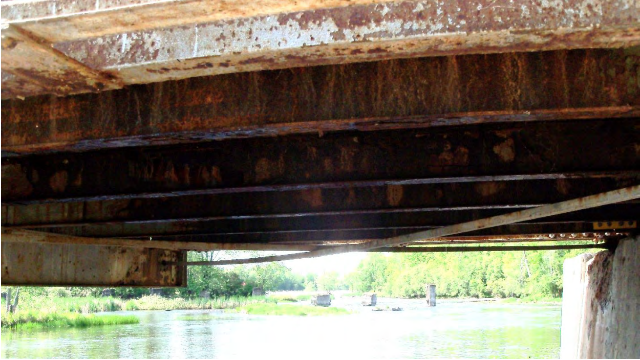
View showing cross bracing and corrosion on girders
