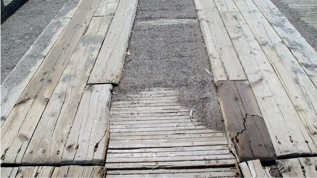
View of deck wearing surface with rot, splits, and checks
