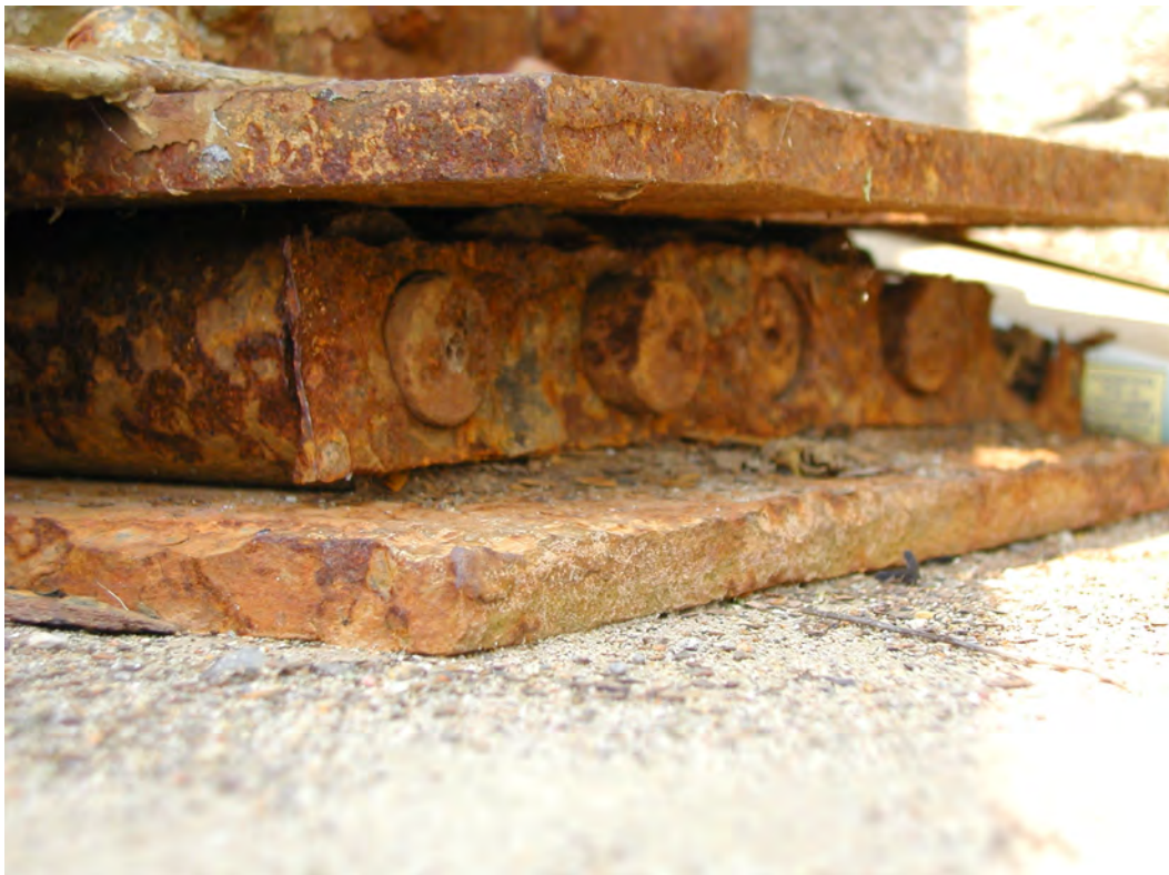
Photograph 22: Detail of deterioration of north roller bearing, West Abutment.
