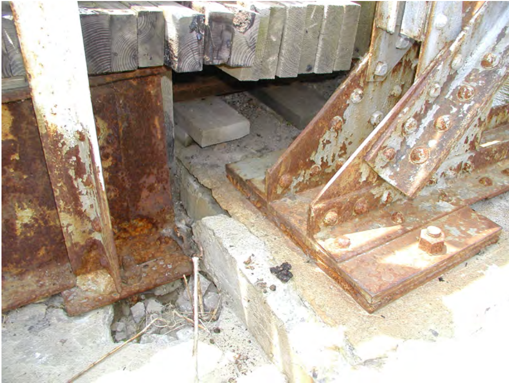
Photograph 25: North bearings at pier. Note undermining of east bearing.
