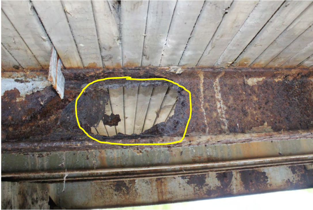
Image 13. Perforation of Approach Stringer 2 after probing
