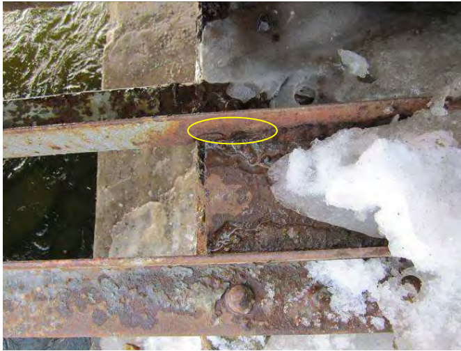
Photograph 4: Moderate pitting vertical leg of bottom chord L0L1
