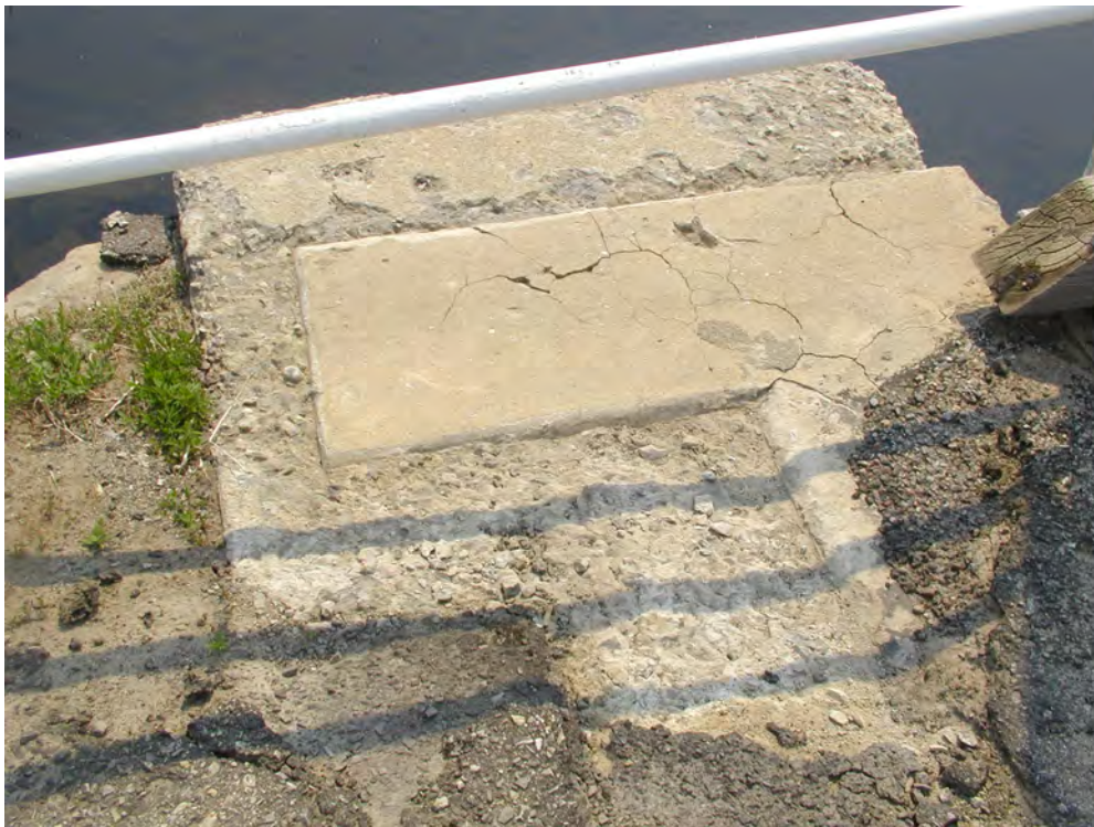
Photograph 32: Detail of top of East Abutment, showing concrete encasement. West Abutment similar.
