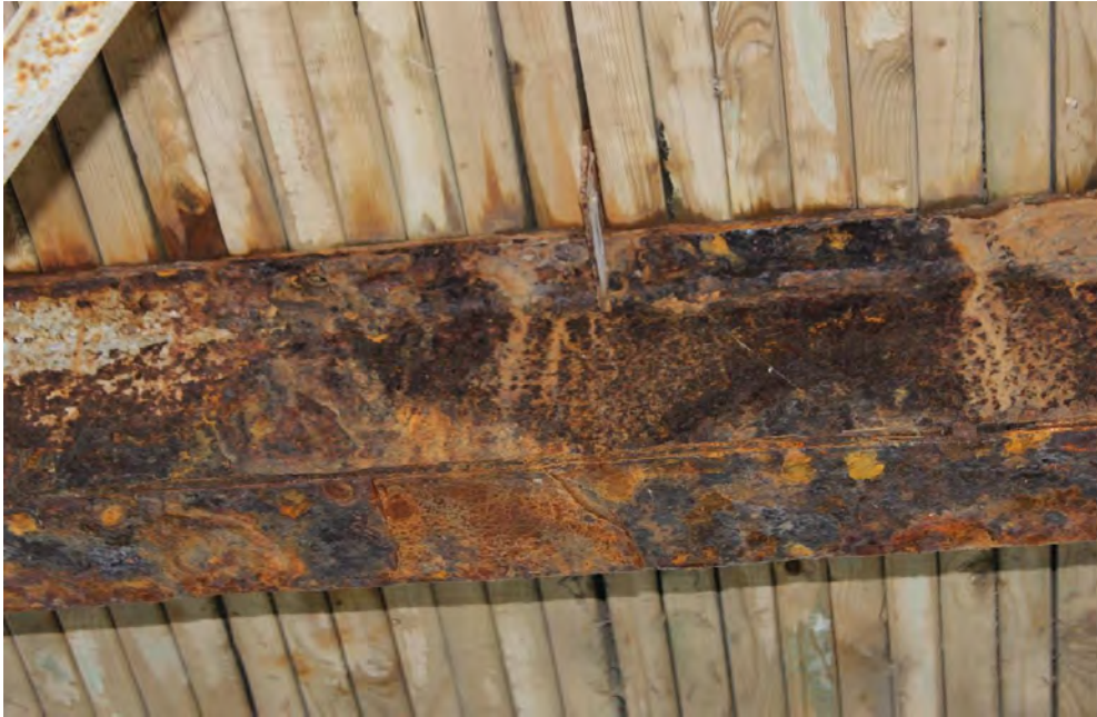
Image 9. South face of Stringer 3 between FB 7 & pier, slab rust and general section loss
