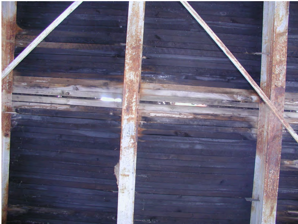
Photograph 12: Creosote is generally missing on timbers in locations of gaps, which have allowed penetration of water.
