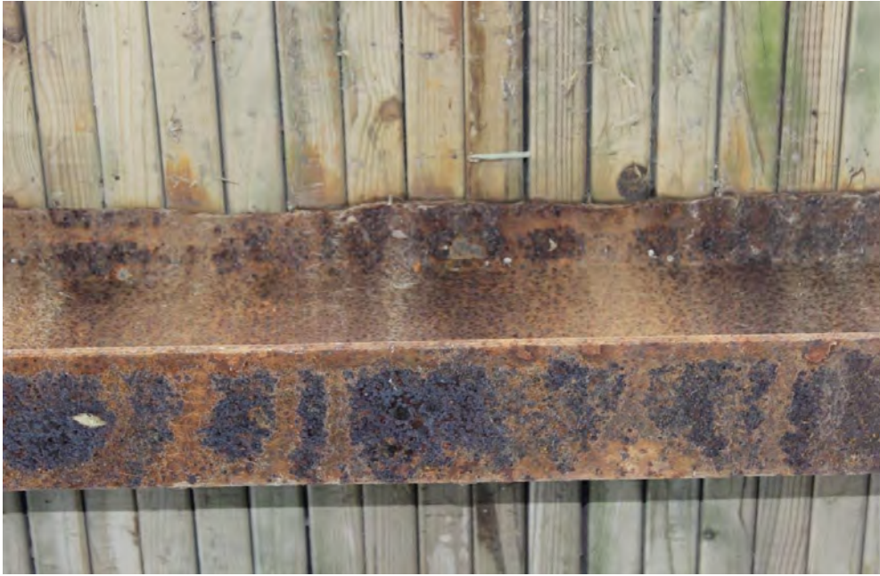
Image 5. Stringer 5, Bay 3 with top flange thinning
