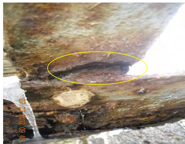
Photograph 3: Severe pitting of horizontal leg of bottom chord L0L1.
