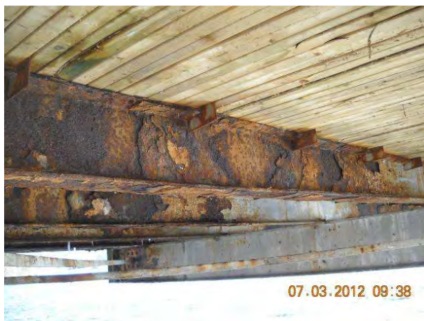
Photograph 2: Typical stringer corrosion in end bay of truss span.
