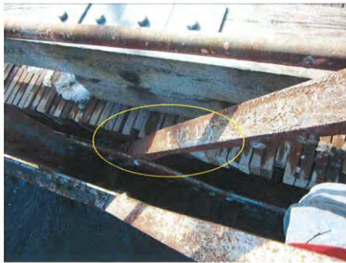
Photograph 6: Twisting of U2L3 (east truss) near L3.
