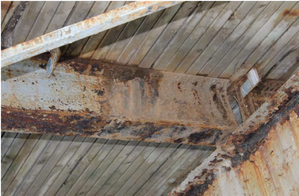
Image 6. Slab rust on north face of web of Stringer 4 adjacent FB 3
