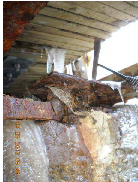
Photograph 5: Severely corroded bottom lateral connection plate at L0
