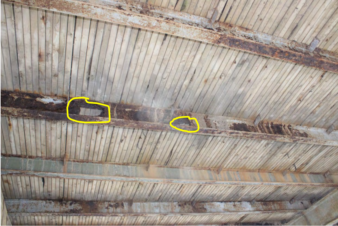
Image 15. General view of west bay of approach span looking downstream. Perforations circled.
