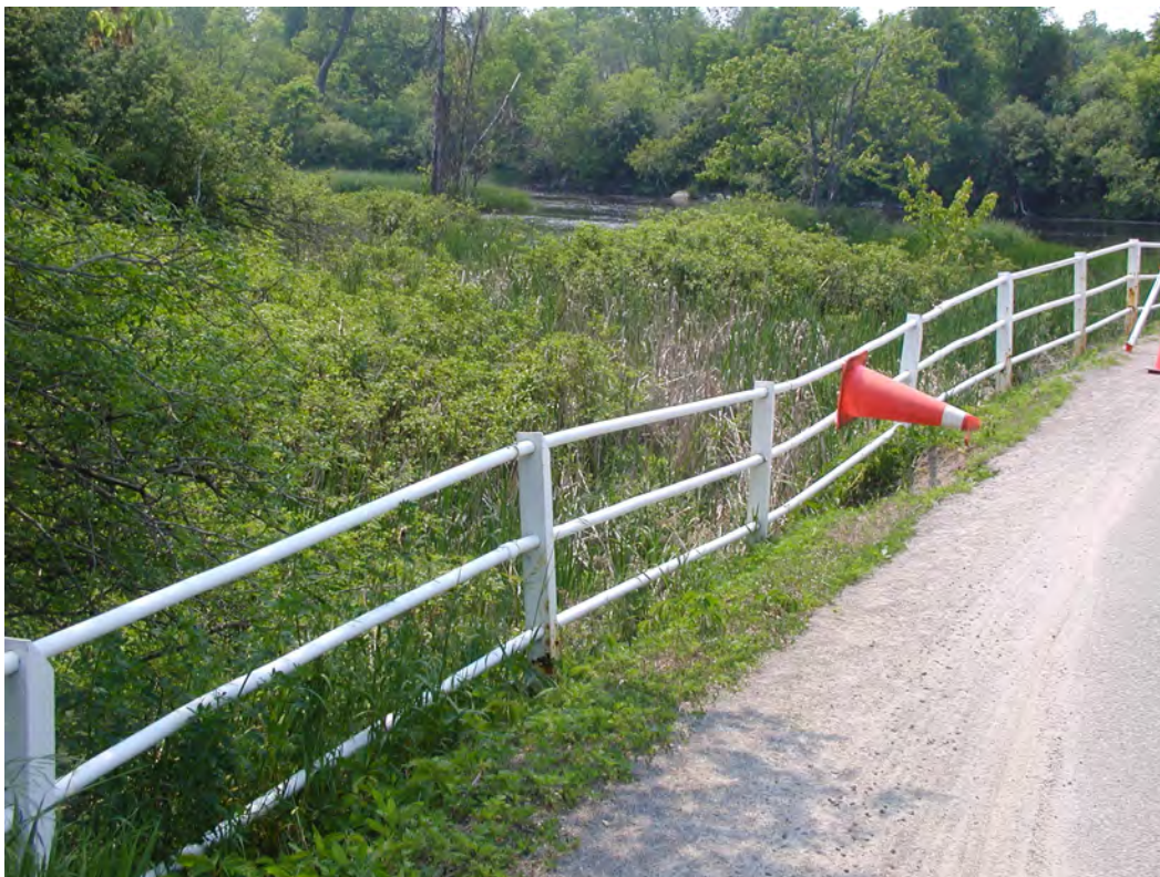
Photograph 34: Deformed railing on south side of east approach retaining wall as a result of slope erosion undermining posts.
