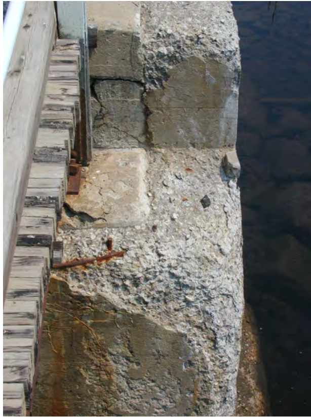
Photograph 31: Deterioration of bearing seat and ballast wall, East Abutment.
