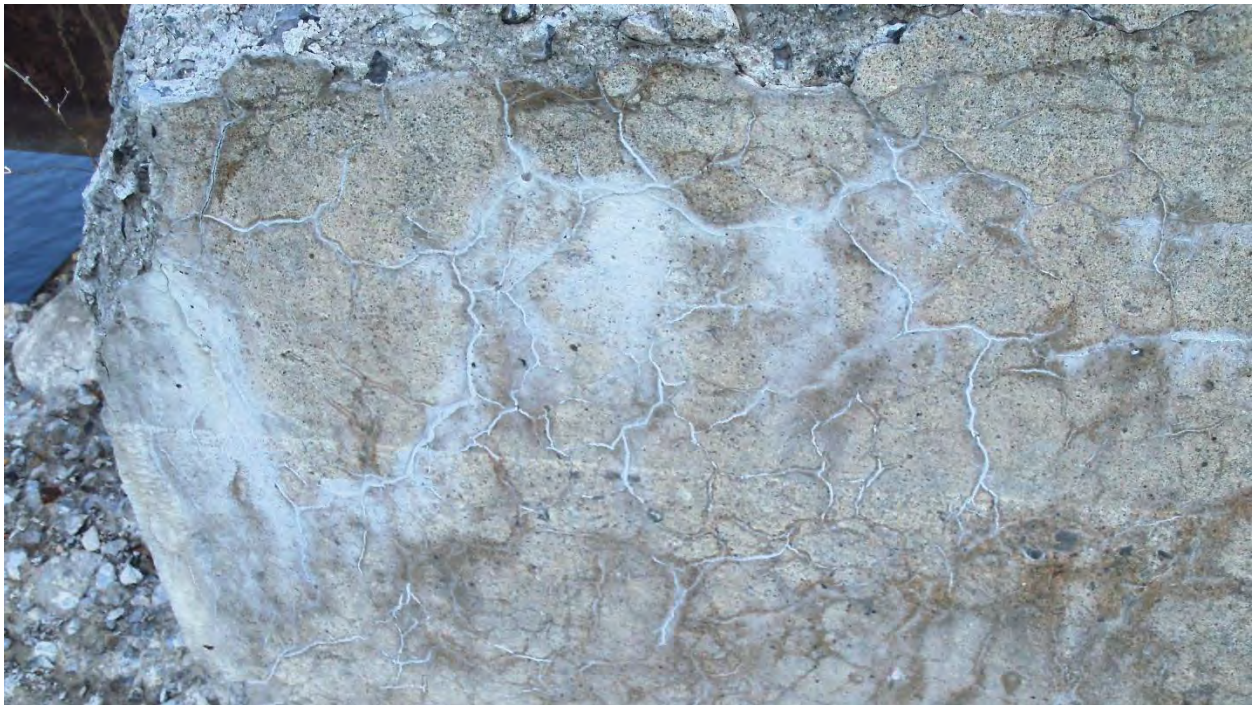
View showing cracking with efflorescence and spalling on the abutment
