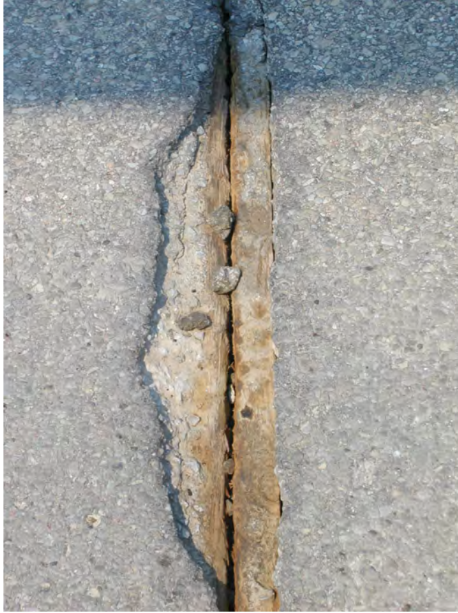
Photograph 9: Detail of deteriorated asphalt showing gap between underlying timbers.
