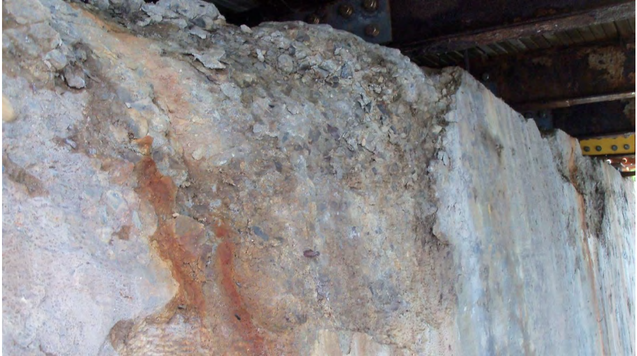
View showing severe spalls and disintegration on abutment
