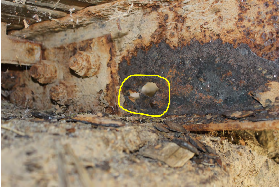
Image 29. Close up of perforated Stringer 2 at east abutment
