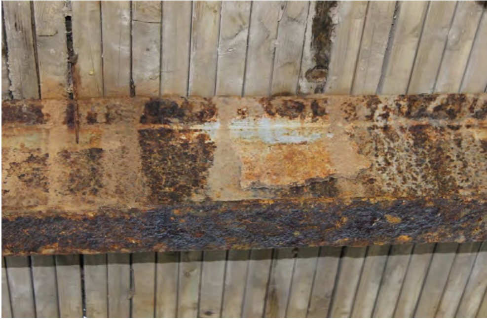
Image 3. Stringer 4 north side adjacent FB 2, slab rust, severe corrosion
