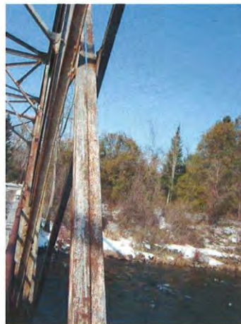
Photograph 7: Buckling of U4L3' (east truss) near mid-height.
