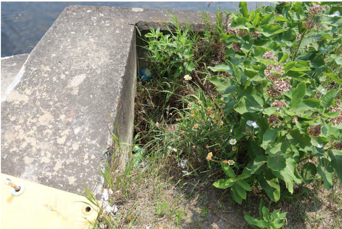
Figure 42: Sinkhole in SW corner
