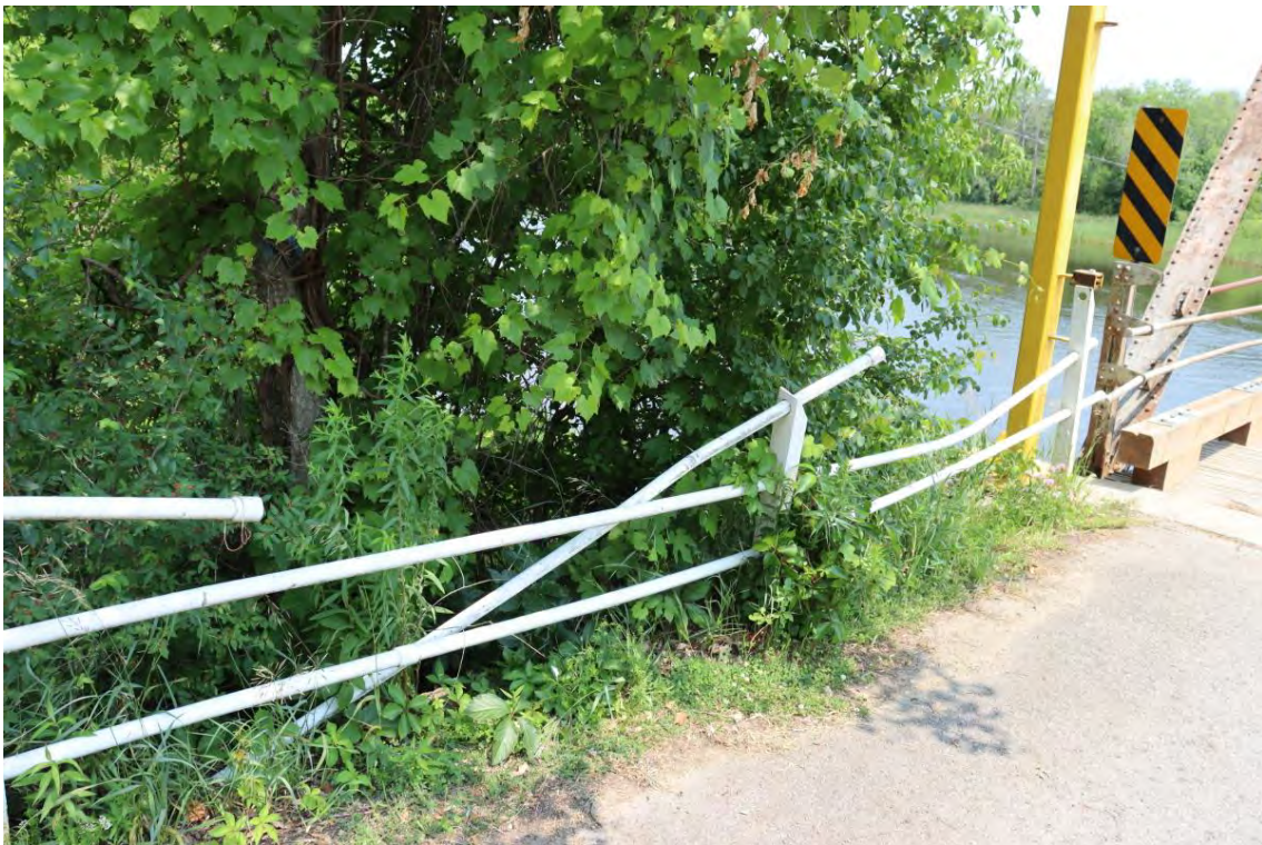
Figure 68: NW damaged approach railing
