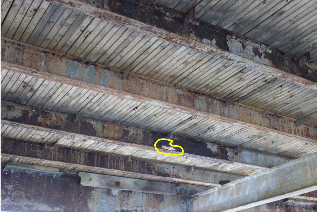
Image 33. East bay of east approach span with perforation in Stringer 2
