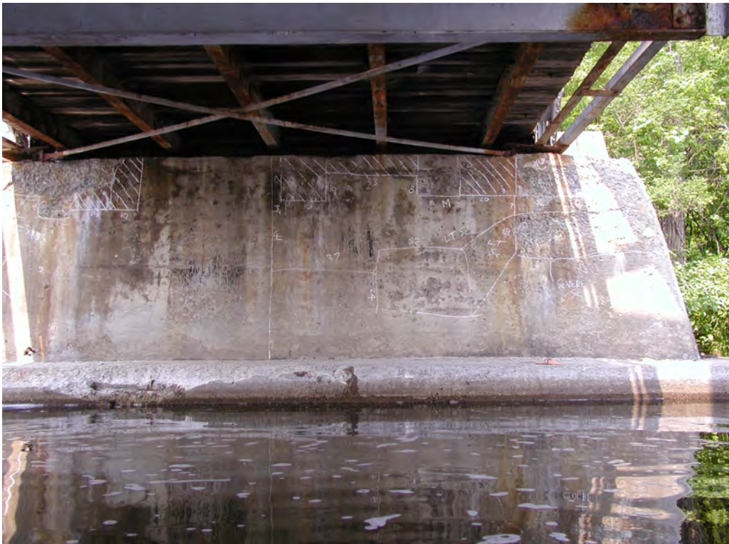
Photograph 26: Face of West Abutment is characterized by extensive scaling, delaminations, and alkali-aggregate reaction. Condition of face of East Abutment is similar.
