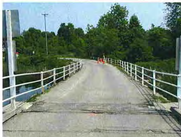
Photograph 3: View of single lane east approach on dry stone retaining walls, looking east.
