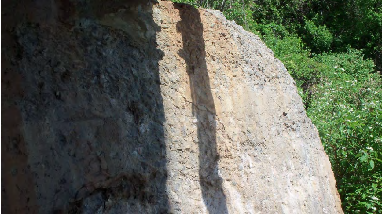
View showing mass spalling and corrosion stains
