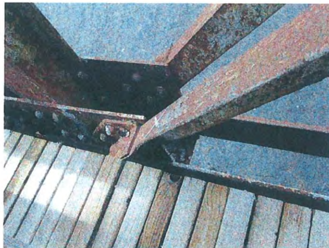
Photograph 2: Deformation in interior angle of U3L4, west truss.
