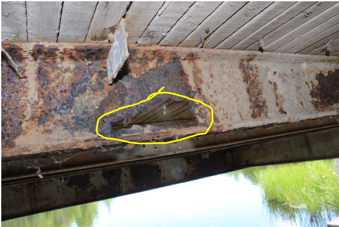
Image 14. Perforation near centre of Approach Stringer 2 west bay.
