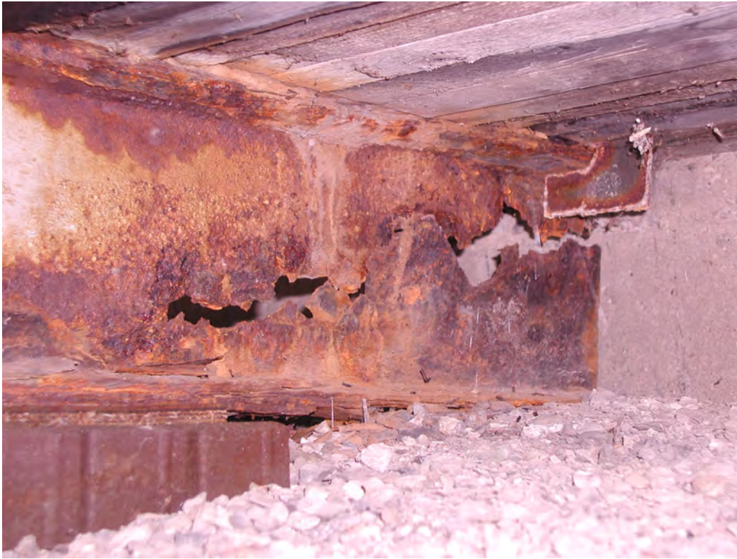
Photograph 19: Very severe section loss in web of middle stringer, West Abutment.
