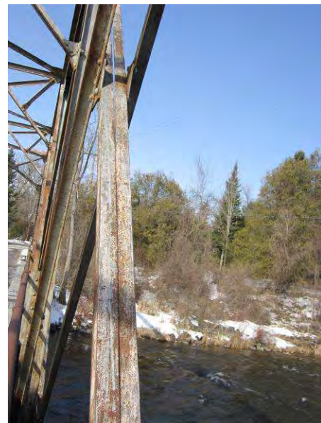
Photograph 7: Buckling of U4L3' (east truss) near mid-height.
