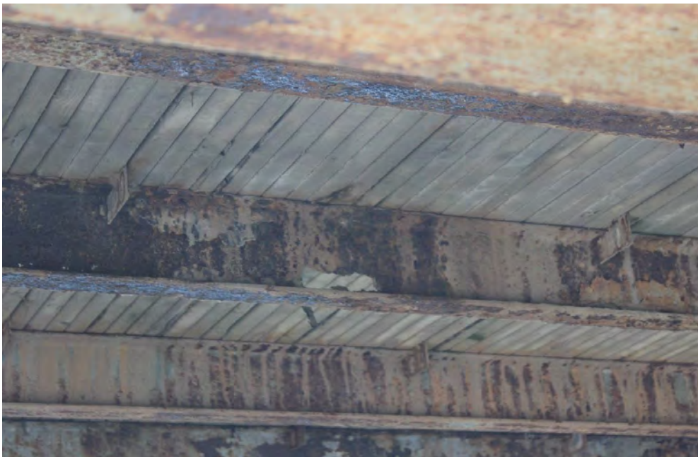
Image 16. Perforated Stringer 2 east end approach span, looking north
