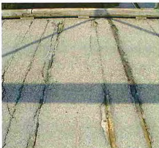
Photograph 4: Deterioration of the asphalt and separation of the deck timbers.
