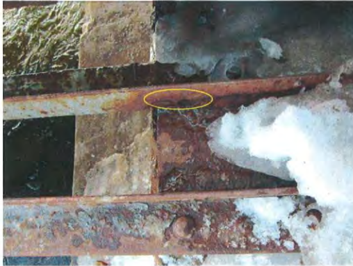
Photograph 4: Moderate pitting vertical leg of bottom chord L0L1
