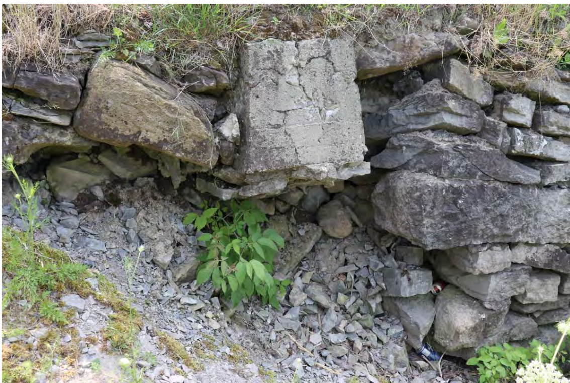
Figure 52: Undercut railing base in north retaining wall east end
