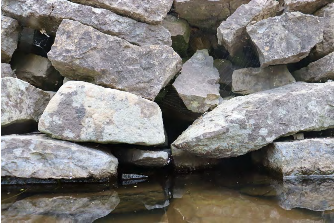
Figure 49: Blocked drainage opening through causeway
