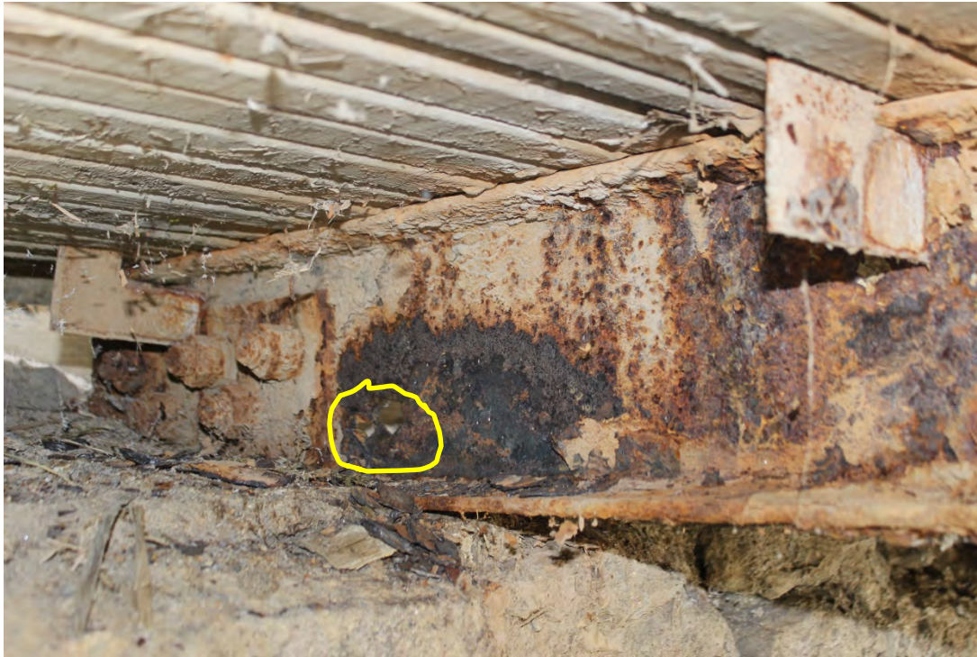
Image 28. Perforated Stringer 2 at east abutment bearing
