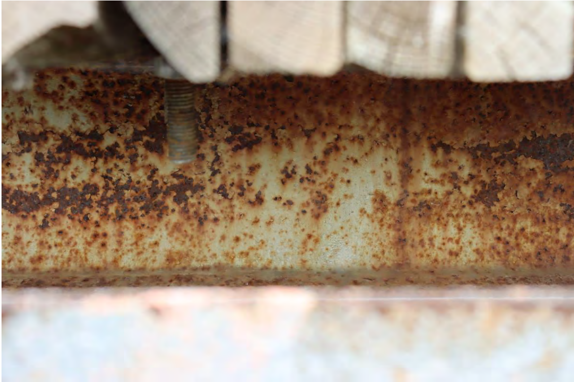
Figure 35: External stringer 1 condition Bay 6
