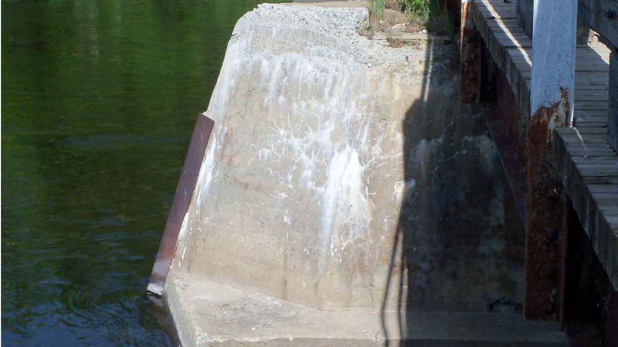
View of pier showing major spalling and efflorescence
