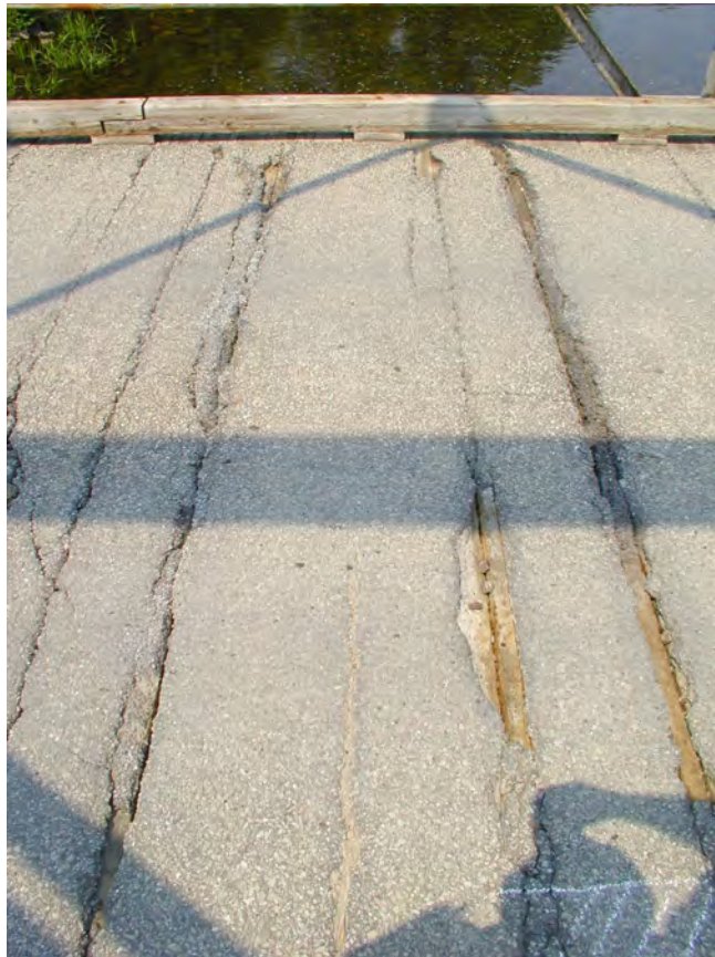
Photograph 8: Detail of asphalt deterioration on timber deck.
