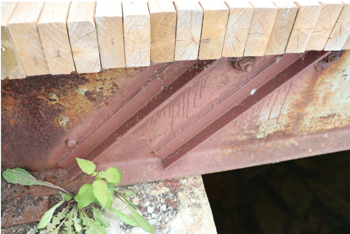
Figure 26: NE girder end web stiffening
