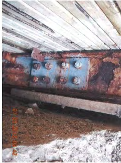
Photograph 9: Displace timber blocking at stringer bearing. Note stringer web repair from 2009 rehabilitation.
