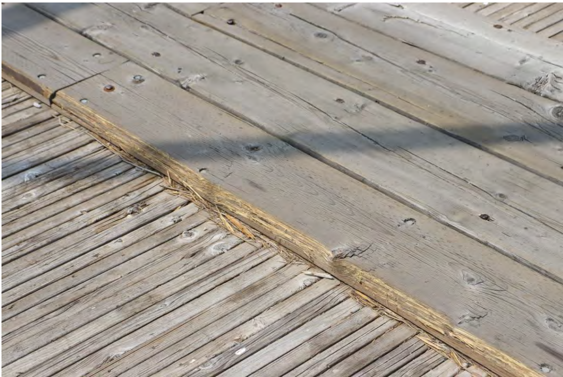
Figure 60: Damaged running boards
