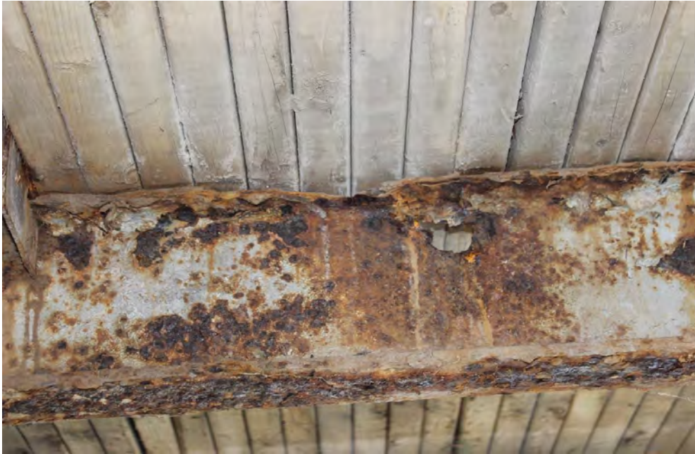
Image 15. Perforated Stringer 4 west end approach span, looking north, severe flange thinning
