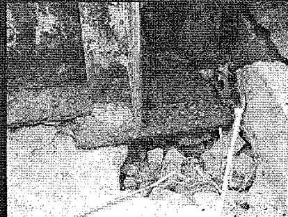
Undermining of south pier bearing
