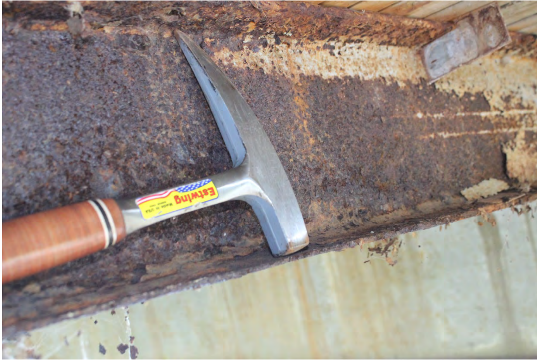
Image 1. Thinning of bottom flange of Stringer 2 in Bay 3
