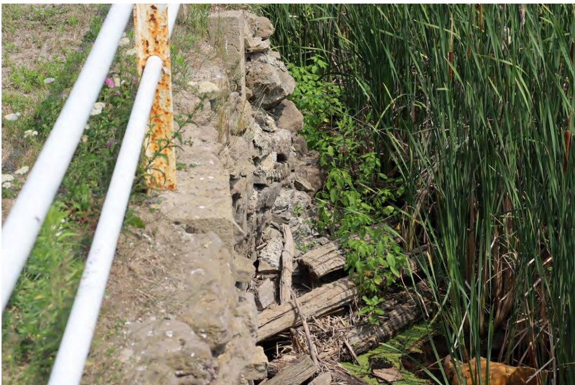
Figure 32: Bulging retaining wall in SE
