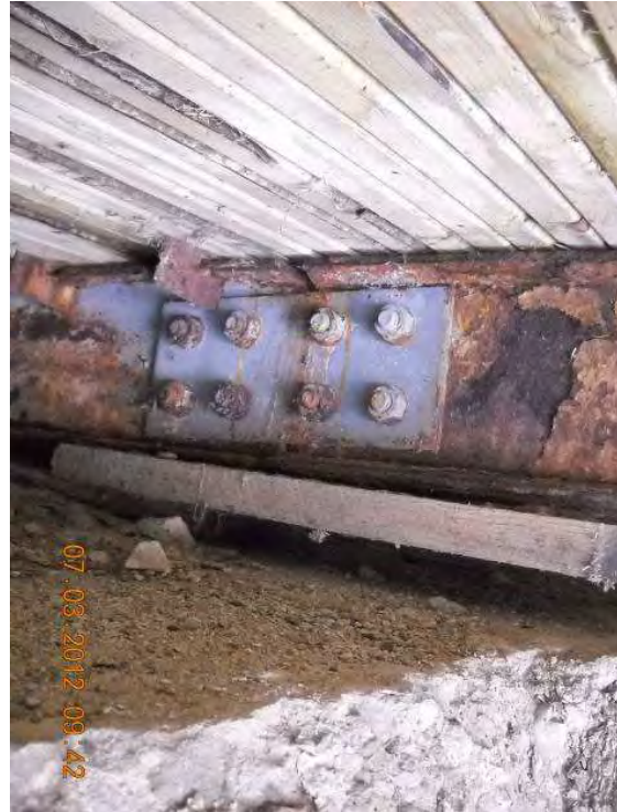
Photograph 9: Displace timber blocking at stringer bearing. Note stringer web repair from 2009 rehabilitation.
