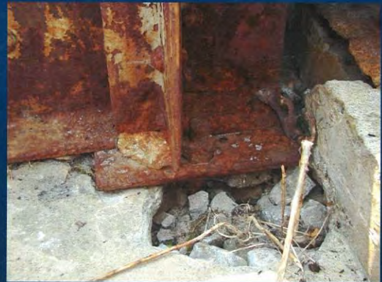
Undermining of south pier bearing
