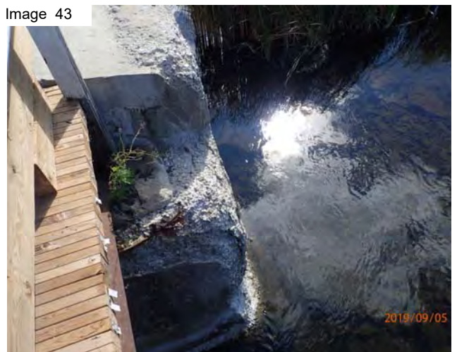
South abutment west corner disintegration
