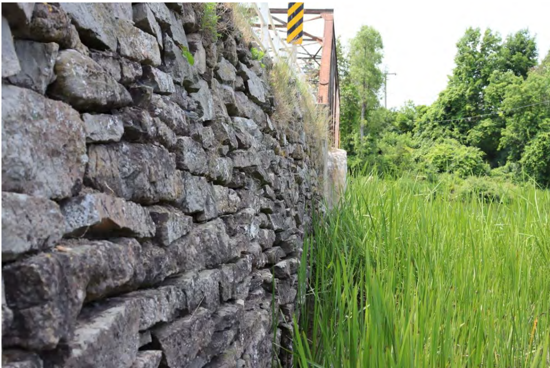
Figure 48: Bulging retaining wall north-east quadrant
