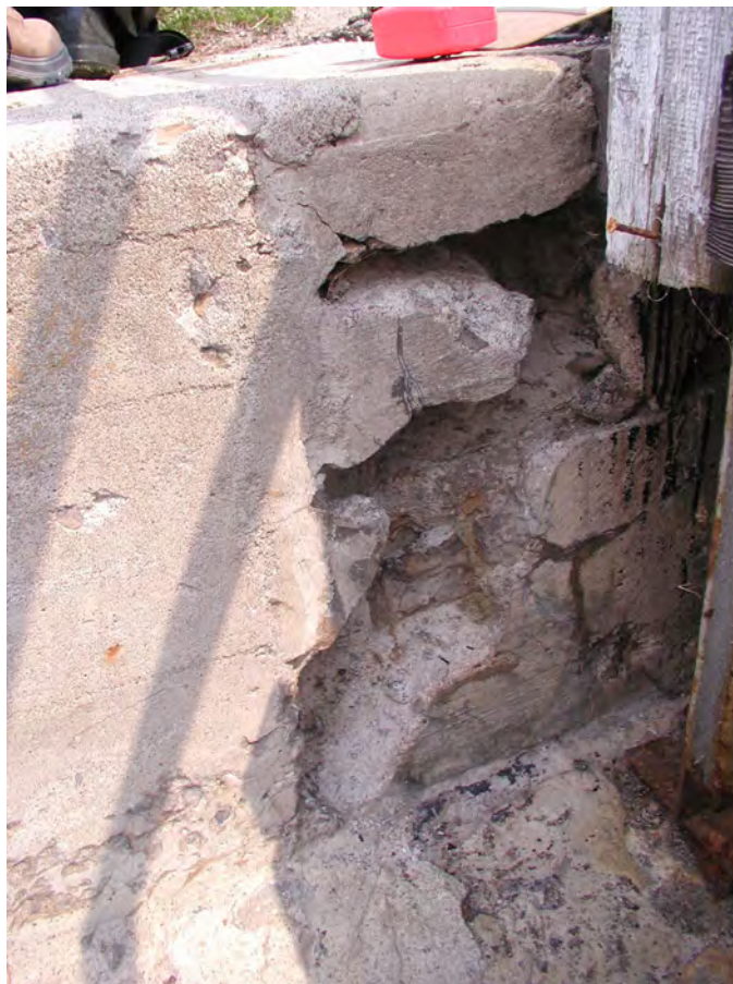
Photograph 30: Detail of deterioration of ballast wall of East Abutment, north side.
