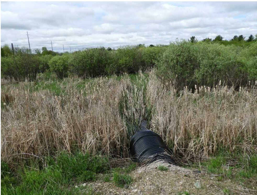
Photo 30: Culvert outlet on Perthmore Street within the Willow Organic Deciduous Thicket Swamp (SWTO2) vegetation community in the southeast end of the study area. 24 May 2019.
